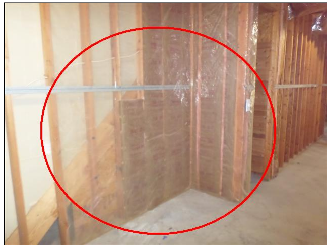
5.0 Item 5(Picture) plastic on walls
