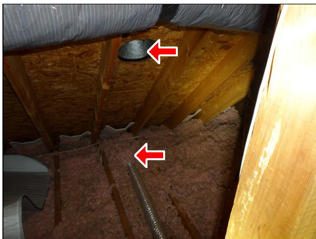
14.1.A Item 1(Picture) pipe disconnected
