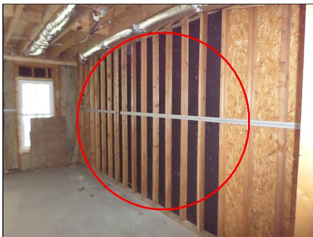
5.0 Item 10(Picture) missing insulation
