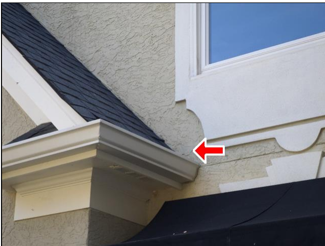
2.1 Item 5(Picture) missing flashing
