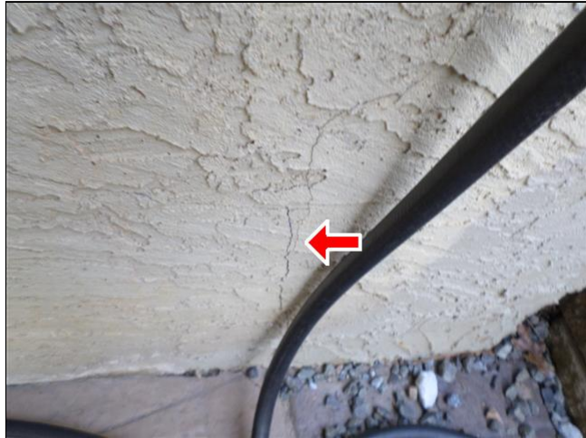
3.0 Item 2(Picture) crack in stucco
