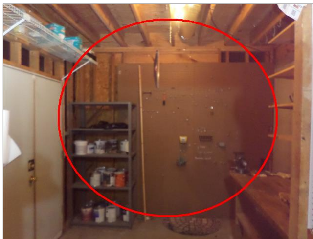
5.0 Item 11(Picture) missing insulation
