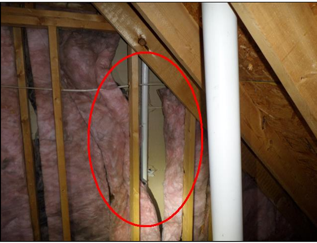
14.2.B Item 1(Picture) loose insulation
