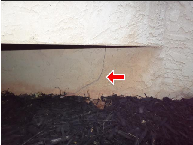
3.0 Item 1(Picture) crack in stucco
