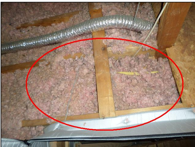
14.4.A Item 2(Picture) missing flooring
