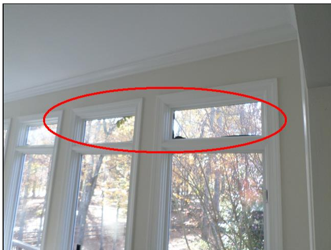
7.2 Item 1(Picture) loose seals
