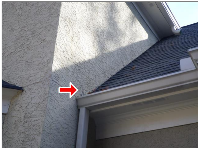
2.1 Item 6(Picture) missing flashing
