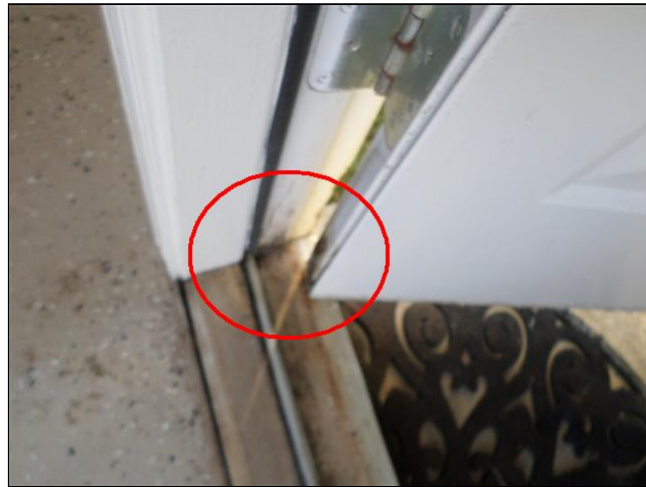
3.0 Item 7(Picture) rot on door and trim
