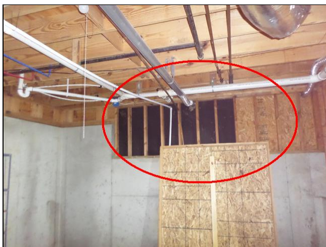
5.0 Item 12(Picture) missing insulation
