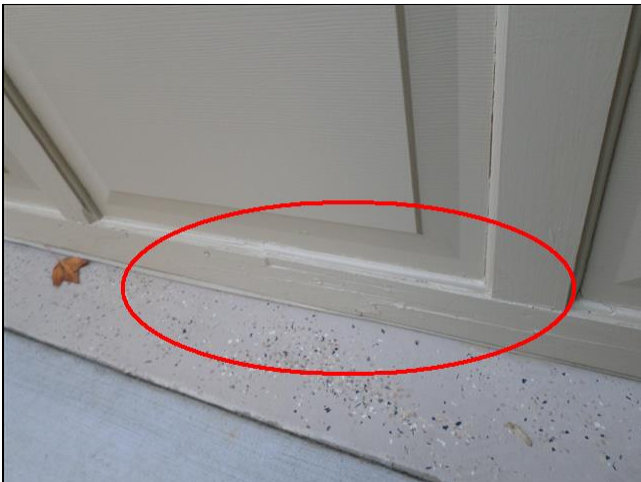
4.3 Item 1(Picture) damage on door panel
