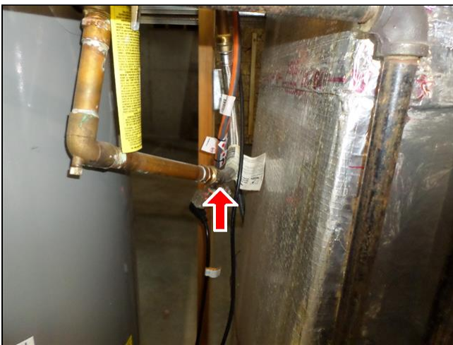
13.0 Item 1(Picture) drain not at lowest point
