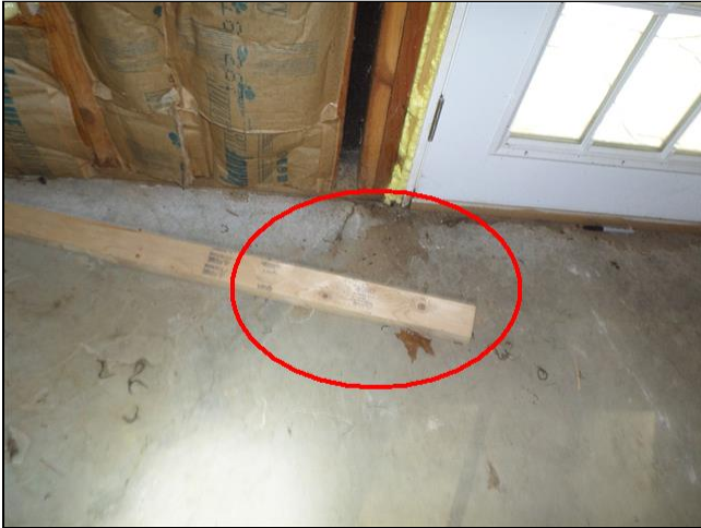
7.3 Item 1(Picture) water spots
