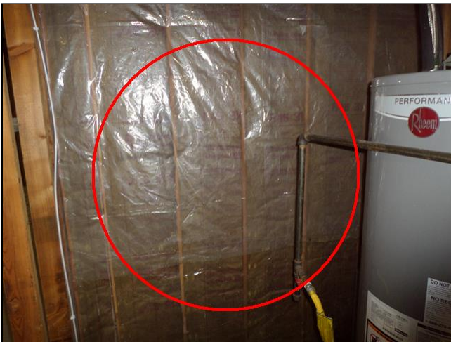
5.0 Item 4(Picture) plastic on walls
