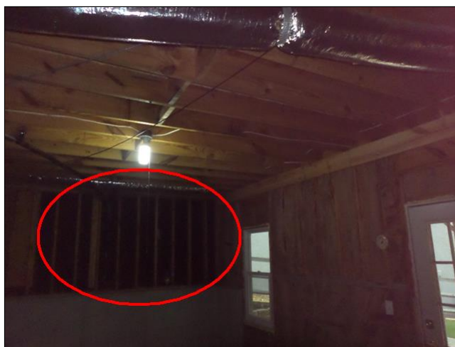
5.0 Item 13(Picture) missing insulation
