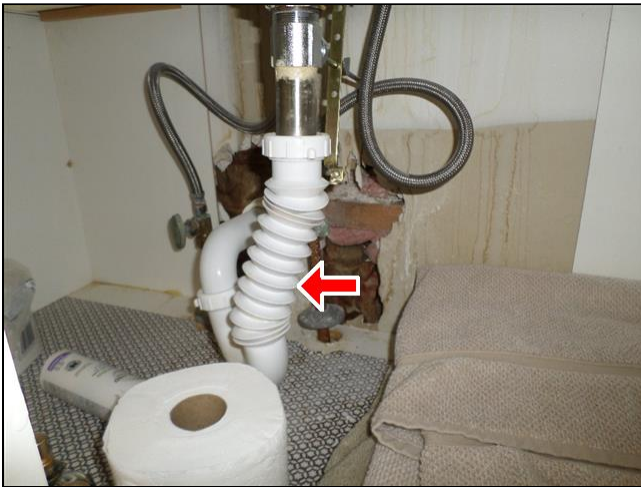
15.6.A Item 1(Picture) accordion drain
