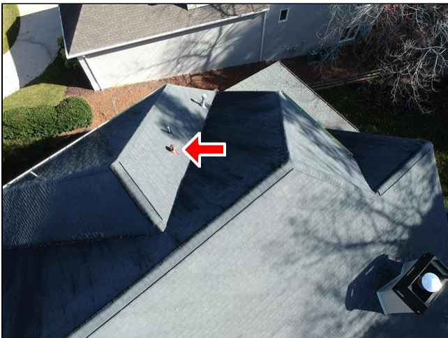
2.1 Item 1(Picture) rust on vent
