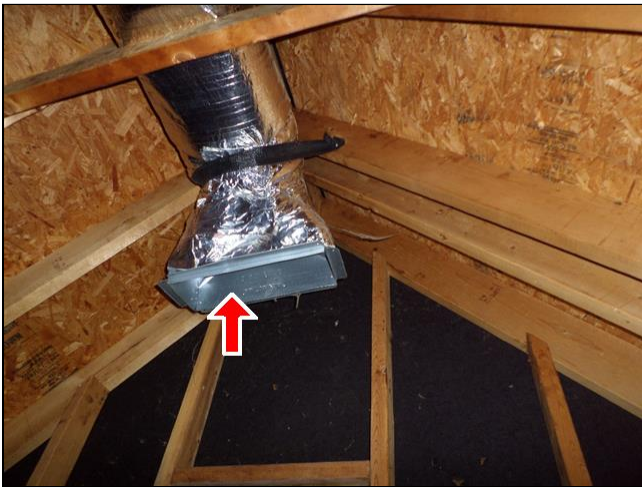
11.3 Item 1(Picture) open duct
