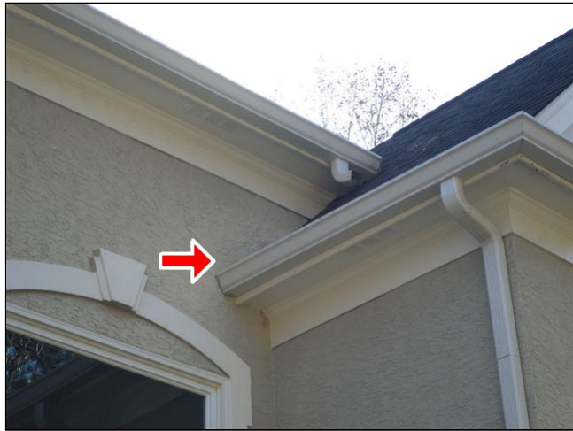
2.1 Item 4(Picture) missing flashing
