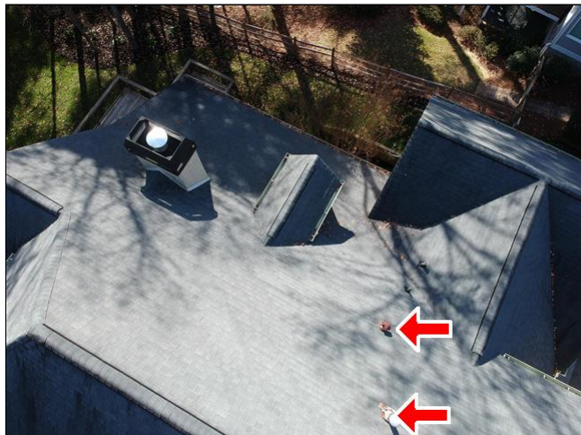
2.1 Item 2(Picture) rust on vents
