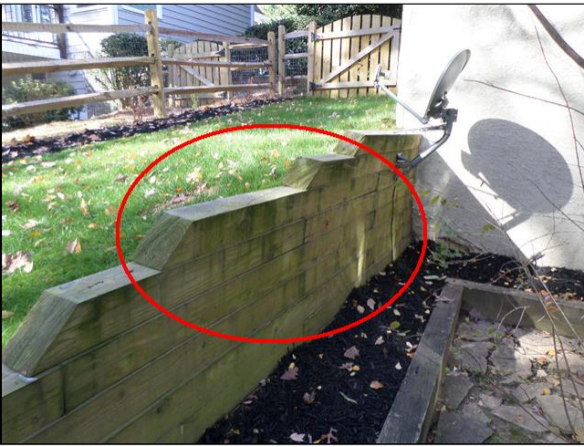
1.9 Item 1(Picture) leaning wall
