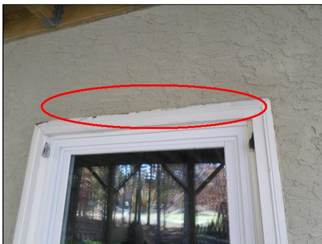
3.1 Item 1(Picture) missing flashing
