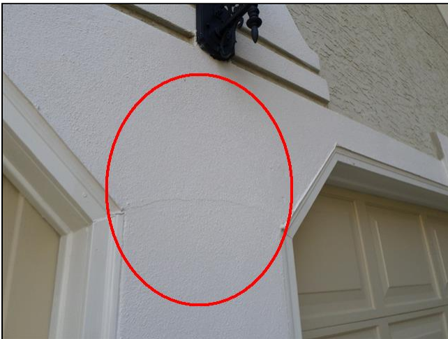
3.0 Item 3(Picture) crack in trim
