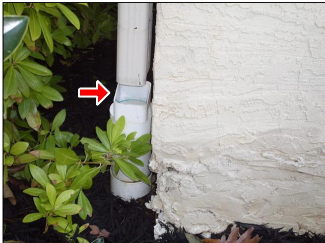
2.3 Item 1(Picture) disconnected pipe
