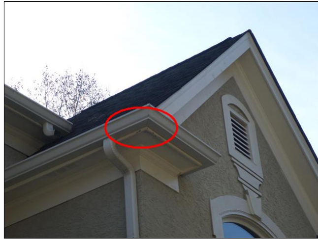
3.0 Item 5(Picture) possible rot
