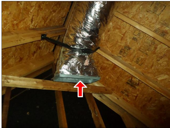
11.3 Item 2(Picture) open duct
