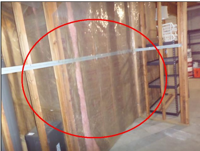
5.0 Item 6(Picture) plastic on walls
