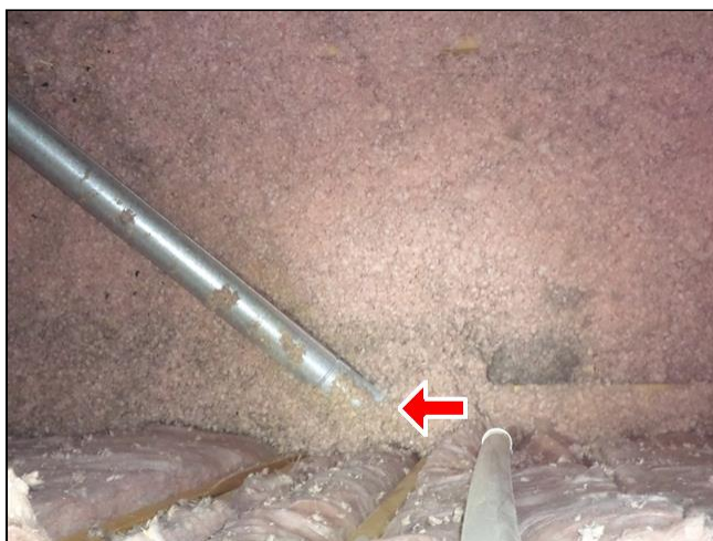
14.2.A Item 1(Picture) vent touching insulation
