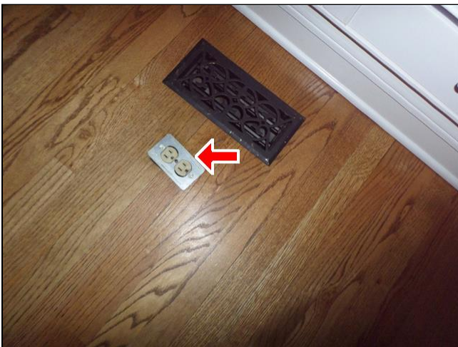
7.5 Item 1(Picture) incorrect cover
