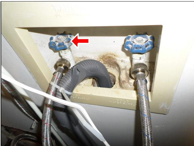
9.0 Item 1(Picture) missing knob
