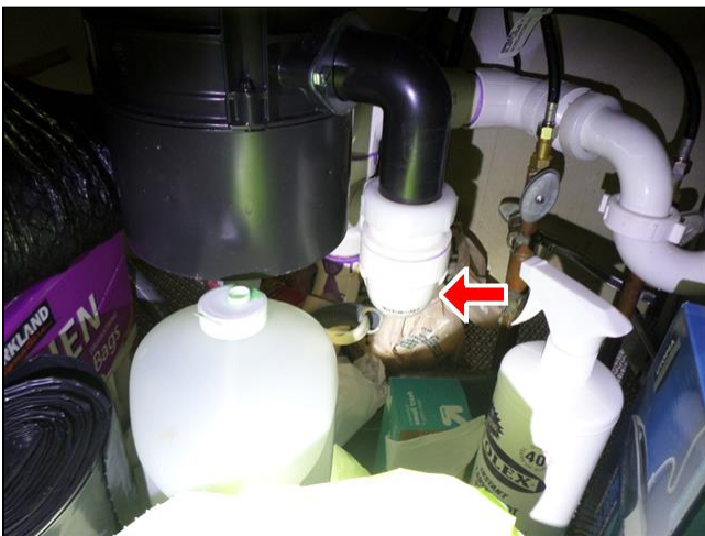
6.8 Item 1(Picture) missing p trap
