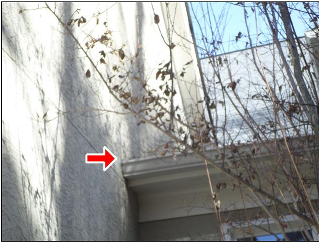
2.1 Item 3(Picture) missing flashing
