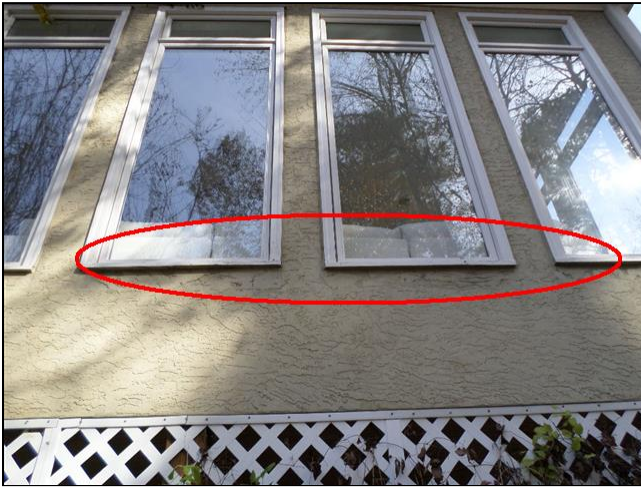
3.0 Item 4(Picture) rotted trim
