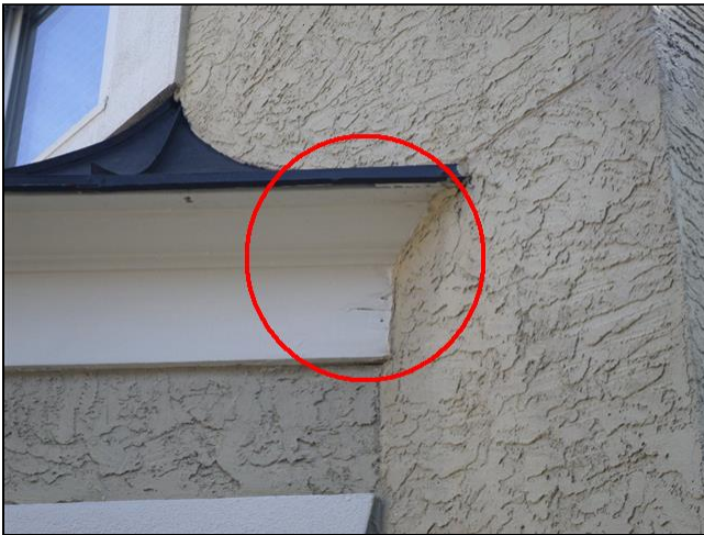
3.0 Item 6(Picture) rotted trim
