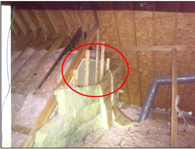
14.2.A Item 2(Picture) loose insulation
