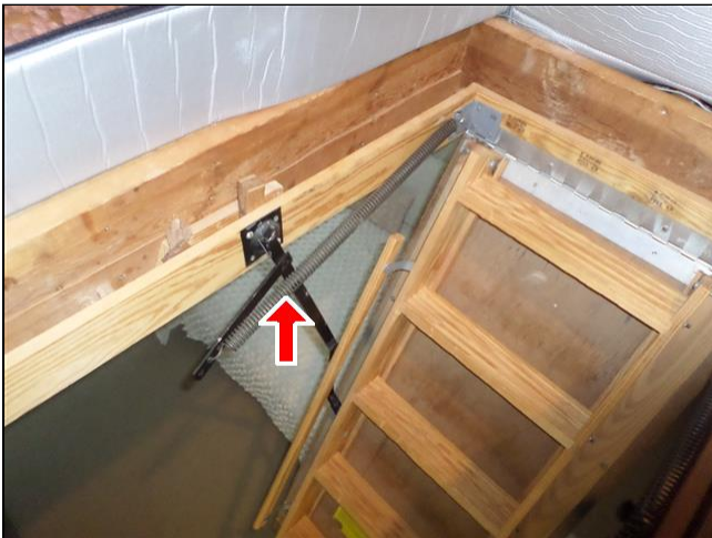
14.4.A Item 1(Picture) loose spring arm
