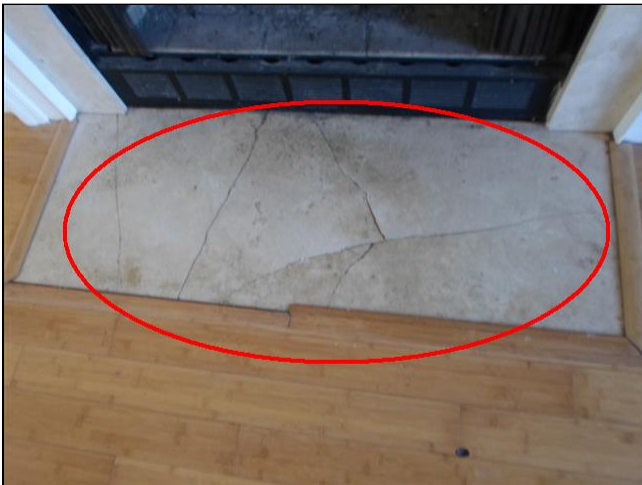
7.7 Item 1(Picture) damaged hearth
