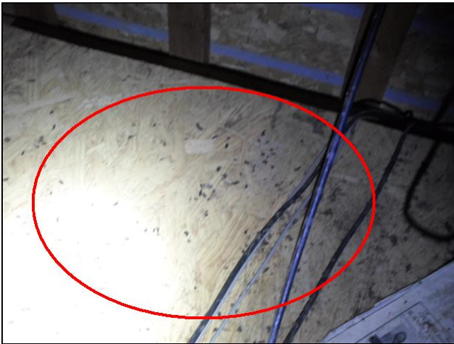
14.5.A Item 1(Picture) rodent droppings
