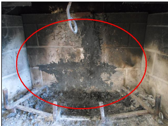
7.7 Item 2(Picture) cracks in fireplace
