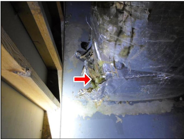
11.3 Item 1(Picture) torn insulation
