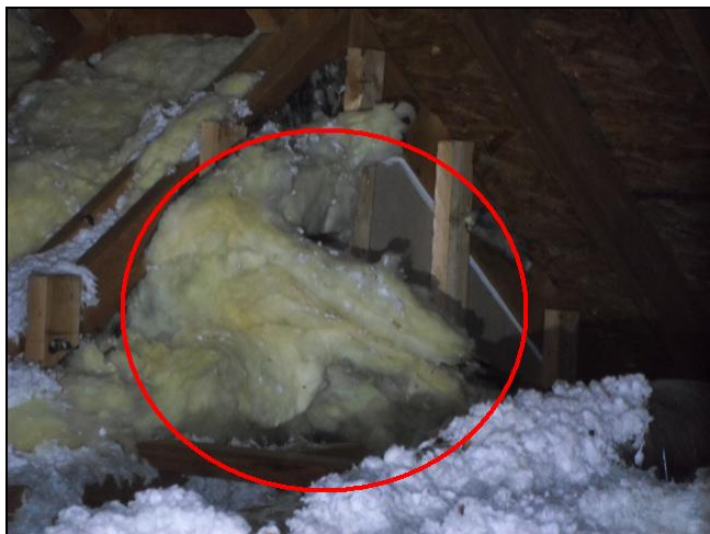
14.2.B Item 1(Picture) loose insulation
