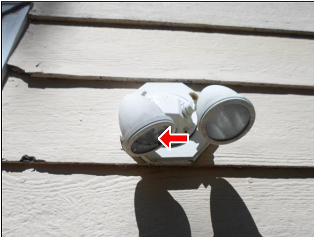
3.4 Item 1(Picture) damaged light
