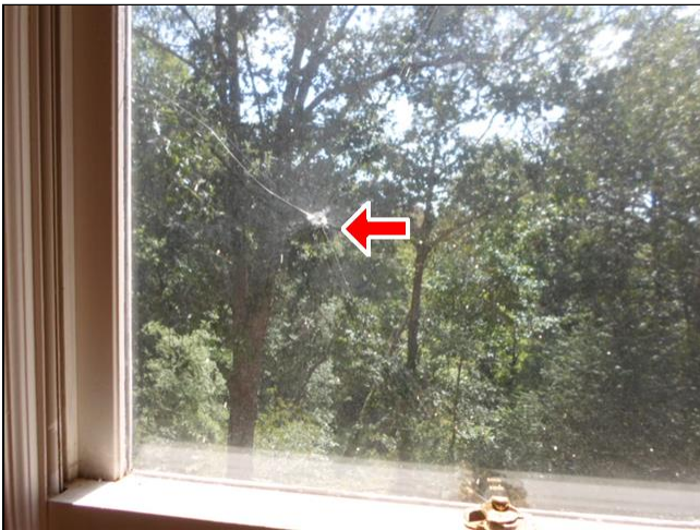
16.2.A Item 1(Picture) broken window
