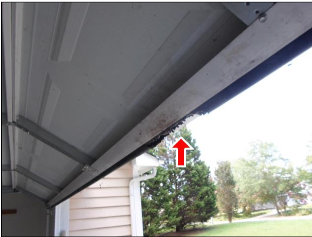
4.3 Item 1(Picture) torn weather stripping
