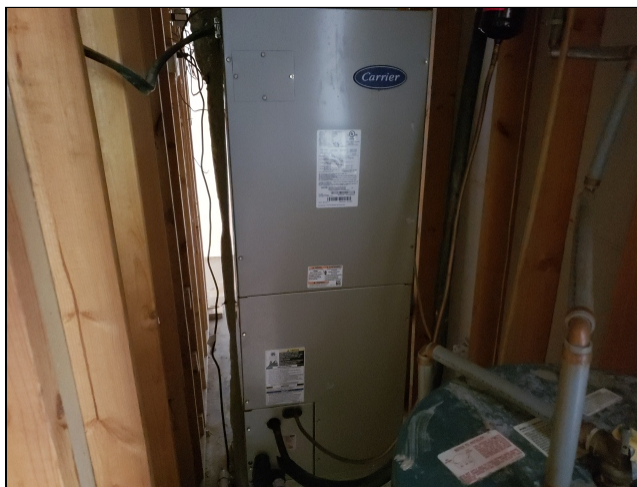
basement heat pump
