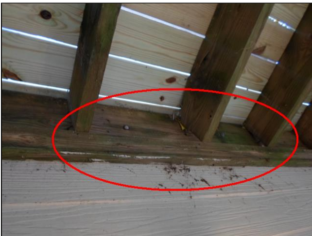
1.3 Item 2(Picture) ledger bowed
