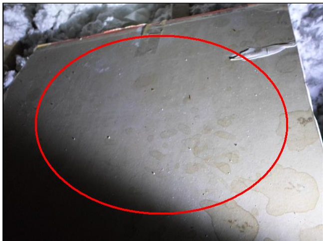
14.4.B Item 1(Picture) missing insulation
