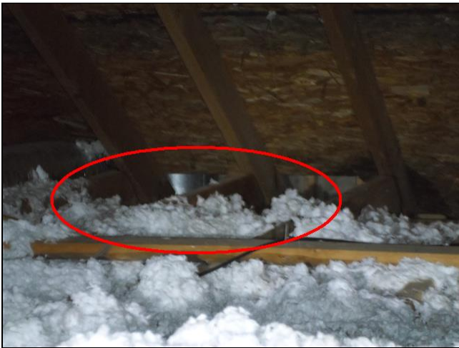
14.0.B Item 1(Picture) missing fire barrier
