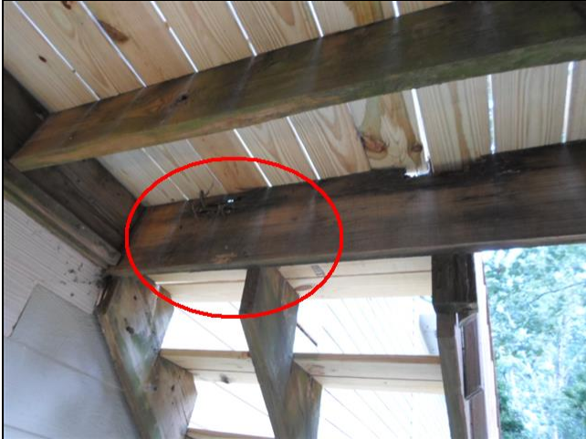
1.3 Item 1(Picture) rot on joist
