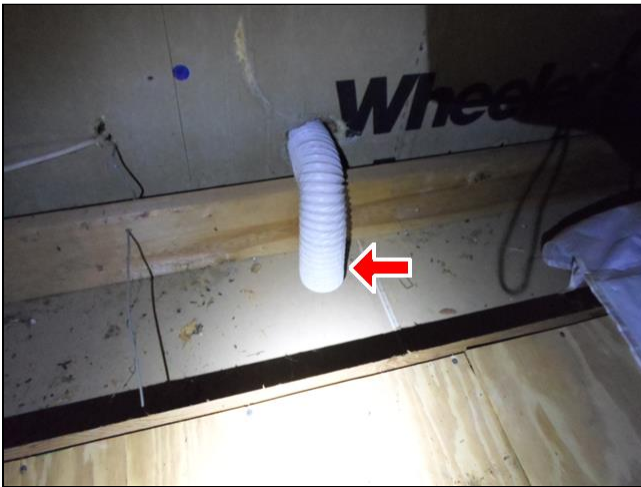
14.1.A Item 1(Picture) fan in attic
