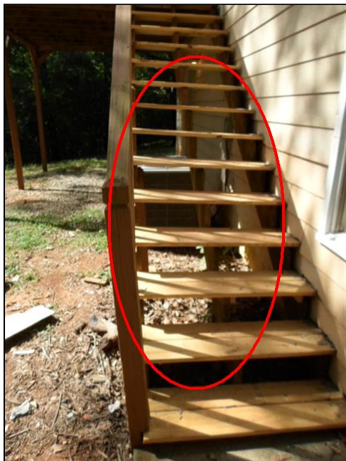
1.5 Item 1(Picture) riser openings too large
