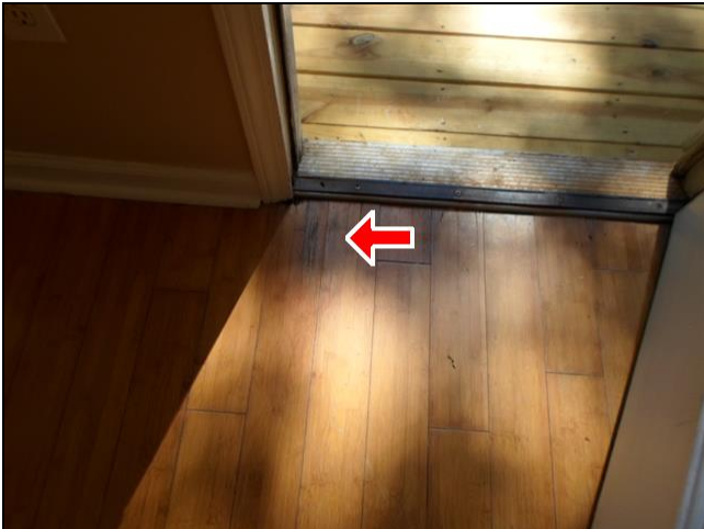
7.3 Item 1(Picture) rot on floor
