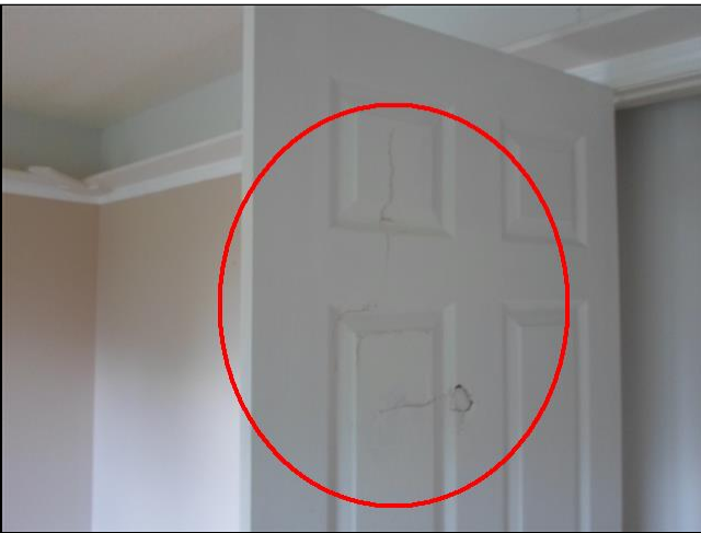
16.4.B Item 1(Picture) damaged door
