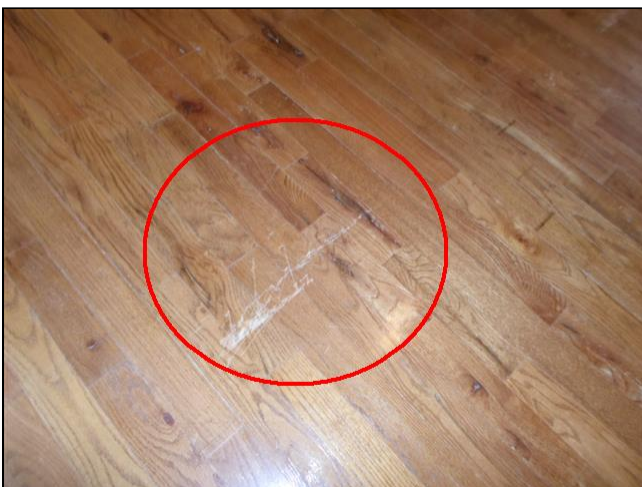
16.3.B Item 1(Picture) damaged floors
