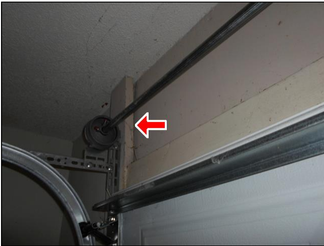
4.3 Item 2(Picture) mount pulling away
