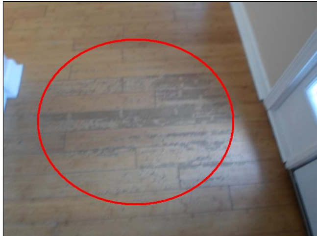
7.3 Item 2(Picture) damaged floor
