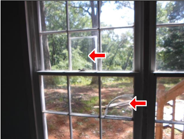
7.2 Item 2(Picture) broken panes
