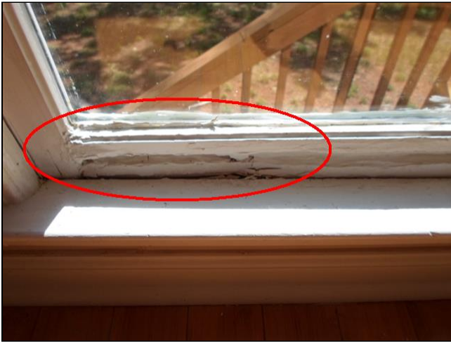
6.2 Item 1(Picture) rot on window
