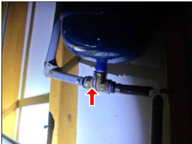
10.1 Item 1(Picture) corrosion on fitting
