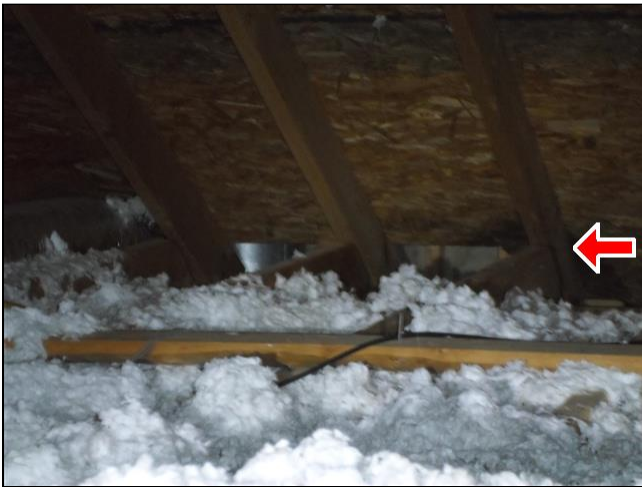
14.0.B Item 2(Picture) water spot
