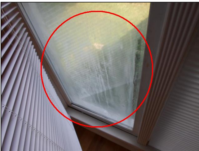
7.2 Item 1(Picture) fogged window
