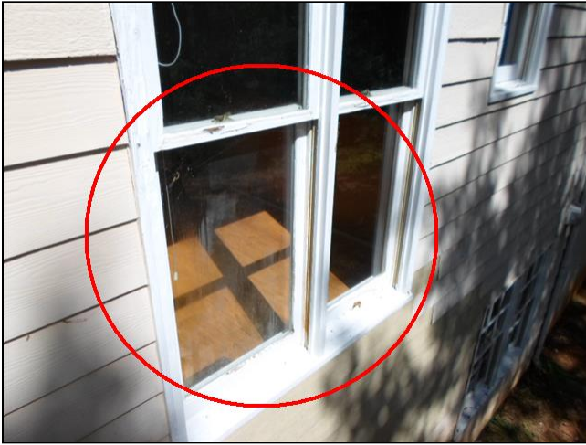
3.0 Item 5(Picture) rotted trim
