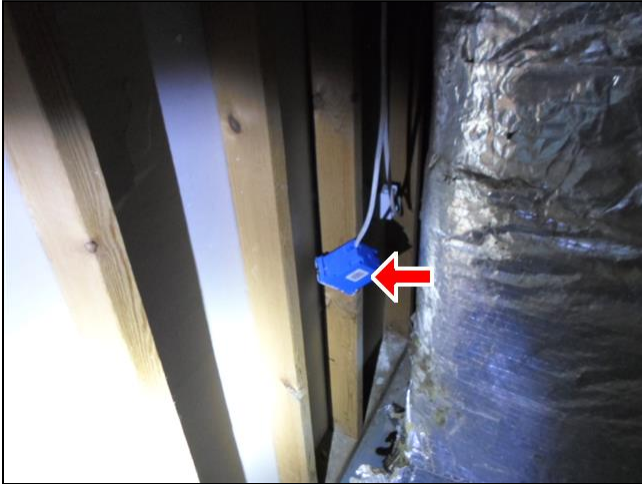
7.5 Item 1(Picture) loose switch
