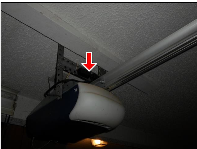
4.4 Item 1(Picture) sensors too high
