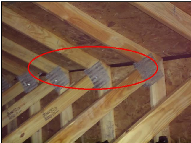
14.1.B Item 1(Picture) small gap
