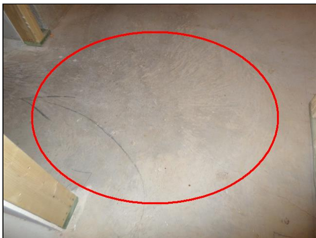
5.0 Item 3(Picture) crack on slab
