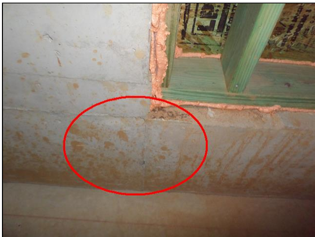
5.0 Item 1(Picture) crack on wall
