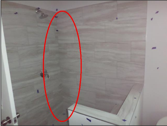
15.7.A Item 1(Picture) open gap
