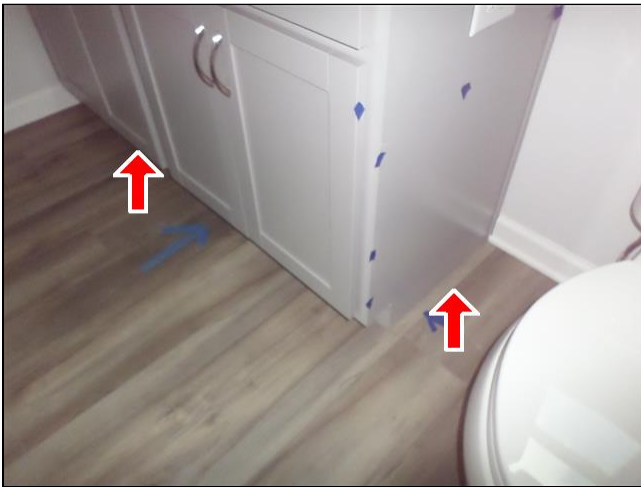
15.5.D Item 1(Picture) missing trim
