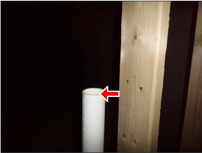
10.2 Item 1(Picture) missing cap
