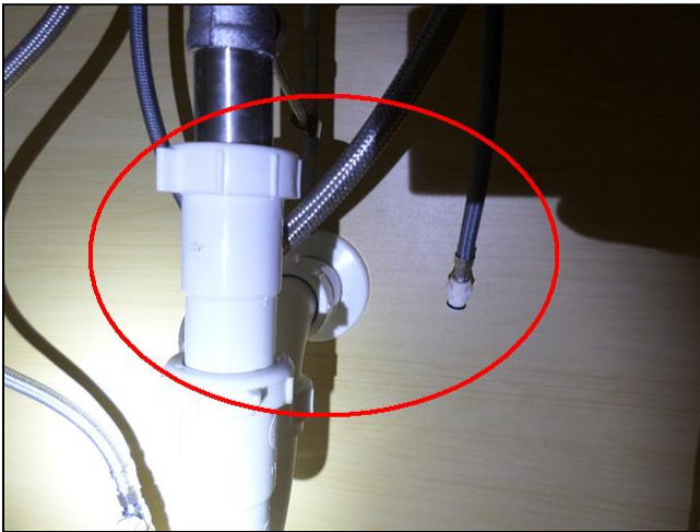
15.6.D Item 1(Picture) water lines not connected
