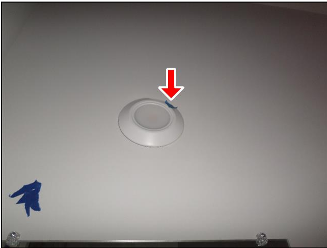
15.3.C Item 2(Picture) loose light
