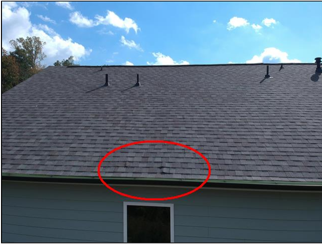
2.0 Item 2(Picture) cupped shingles
