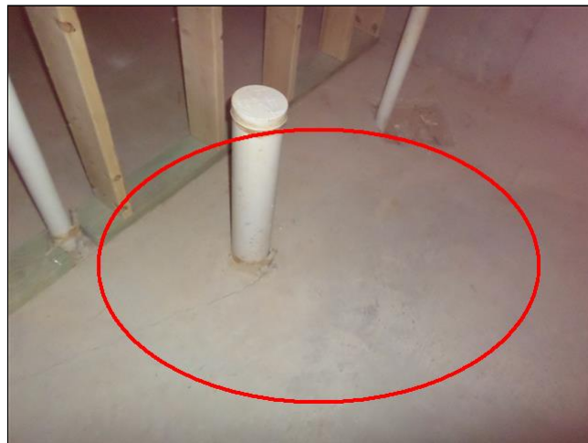
5.0 Item 2(Picture) crack on slab
