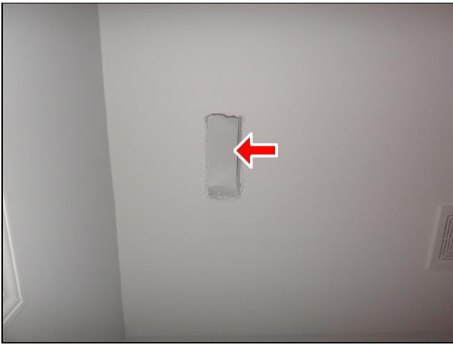
15.3.C Item 1(Picture) missing vent
