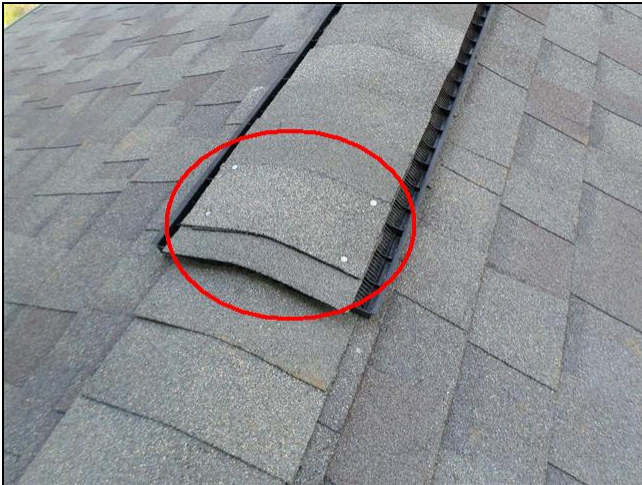
2.1 Item 1(Picture) exposed nails
