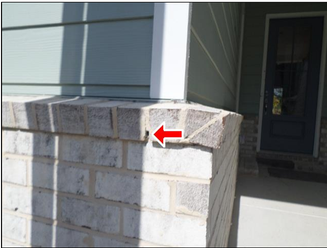
3.0 Item 1(Picture) open joint
