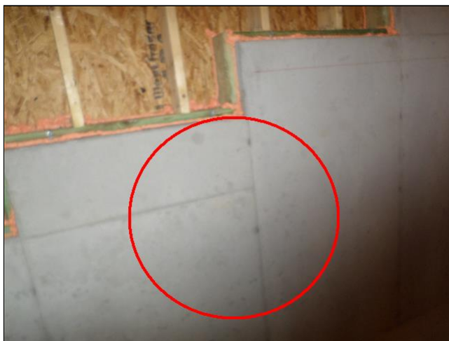
5.0 Item 4(Picture) crack on wall
