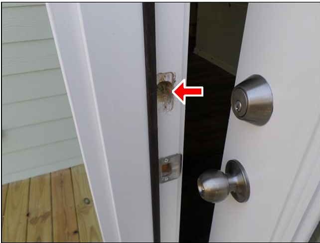
3.2 Item 1(Picture) missing strike plate
