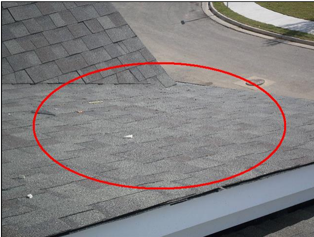
2.0 Item 1(Picture) debris on roof
