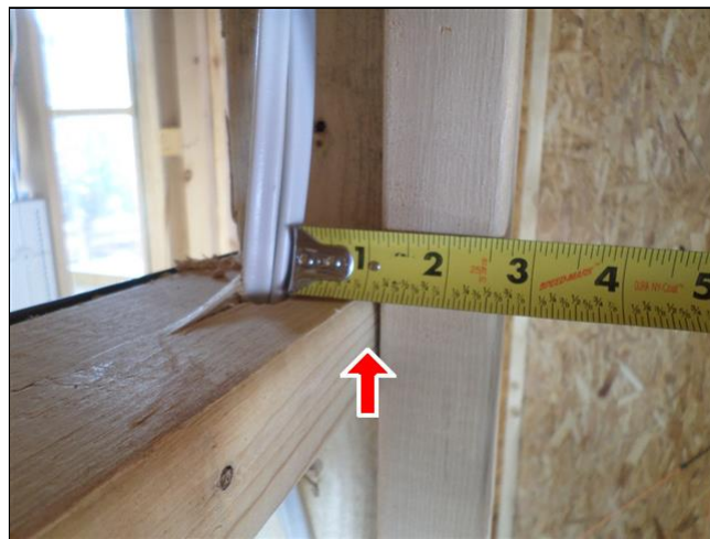
2.8 Item 2(Picture) missing plate in right hallway
