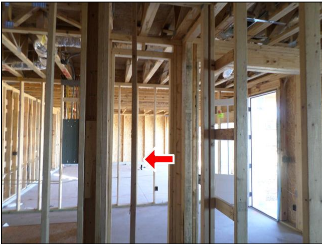
2.3 Item 11(Picture) bowed stud on right closet wall
