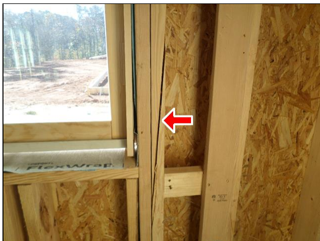
2.3 Item 9(Picture) splitting on right laundry room wall
