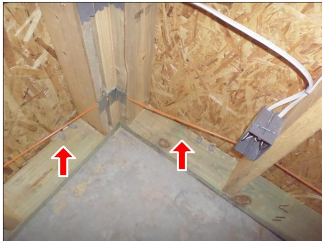
2.3 Item 7(Picture) missing bolts in living room
