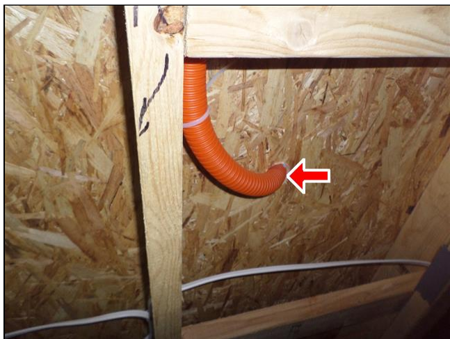
2.3 Item 1(Picture) missing sealant
