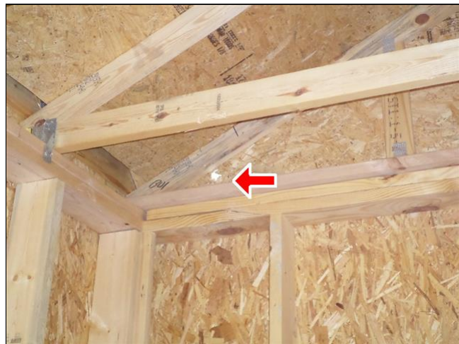
3.0 Item 6(Picture) damaged sheathing on left wall in front left bedroom
