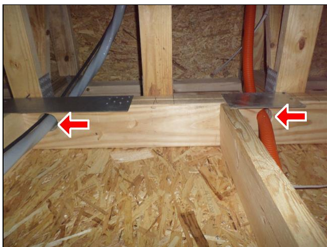
2.3 Item 3(Picture) missing sealant
