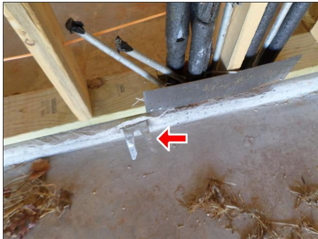
2.3 Item 14(Picture) missing nails
