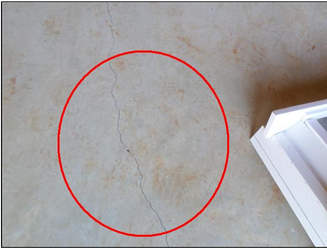
2.5 Item 1(Picture) crack in slab
