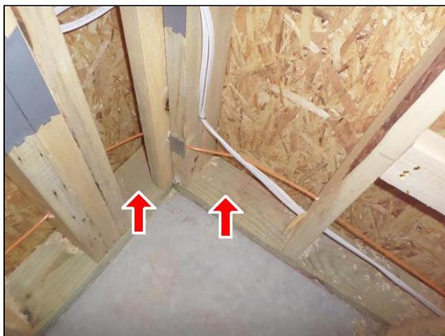
2.3 Item 8(Picture) missing bolts in living room
