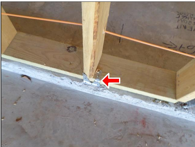
2.3 Item 15(Picture) missing nails
