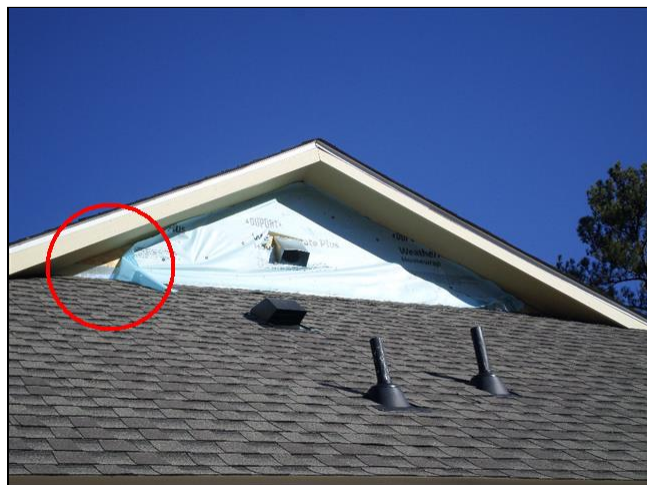
3.0 Item 1(Picture) loose house wrap
