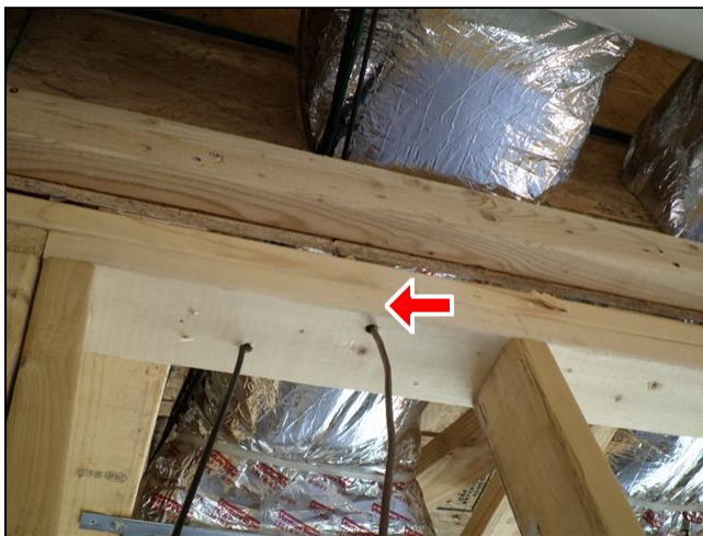
2.8 Item 1(Picture) missing plate on left family room wall
