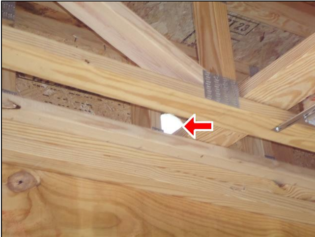
3.0 Item 3(Picture) hole on rear master bedroom wall
