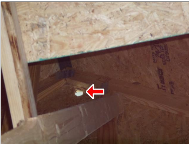
3.0 Item 5(Picture) damaged sheathing on front wall in front left bedroom
