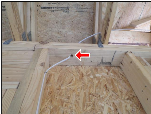
2.7 Item 2(Picture) missing sealant
