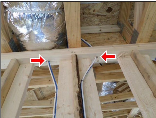
2.7 Item 1(Picture) missing sealant
