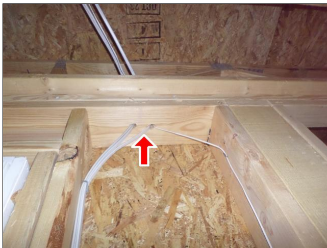
2.3 Item 2(Picture) missing sealant
