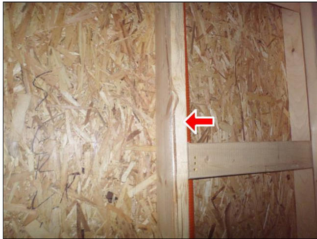
2.3 Item 12(Picture) damaged stud on left living room wall
