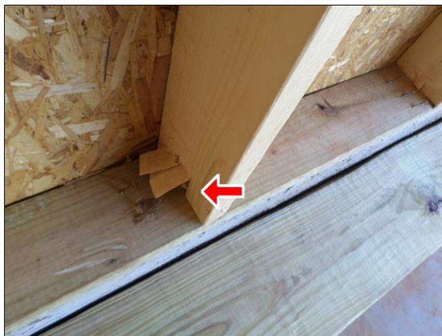
2.3 Item 10(Picture) damaged stud on right garage wall
