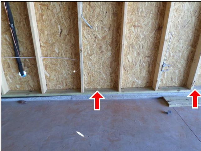
2.3 Item 6(Picture) missing bolts on right garage wall
