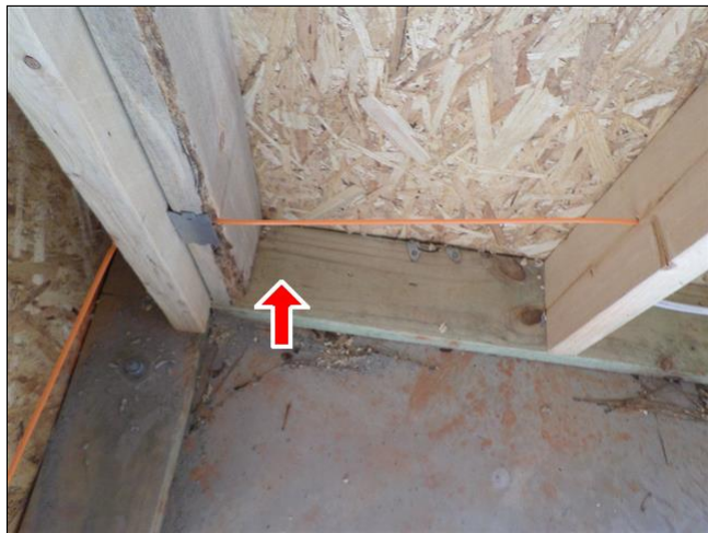
2.3 Item 5(Picture) missing bolt on rear master bedroom wall
