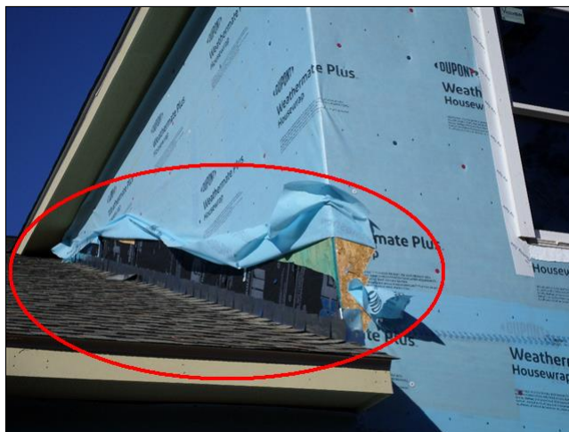
3.0 Item 2(Picture) loose house wrap
